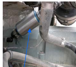
Typical Diesel Installation for closed systems. Note the minimum 45 degree angle from vertical.
